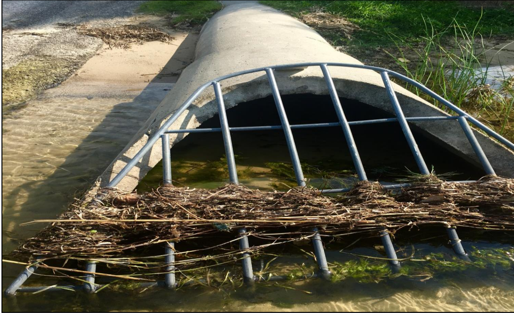
Figure 3. An outlet structure that receives water from Barron Lake, Cass County, Michigan (RLS, 2017).
